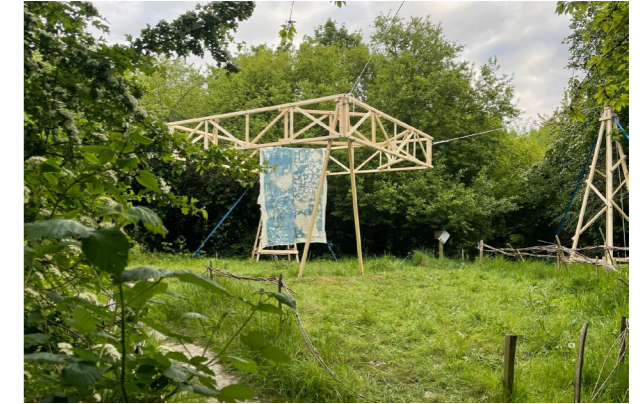
PITCH under construction. Stave Hill Ecological Park, Rotherhithe, London. 28/04/2022. Cyanotype with Art Assassins, South London Gallery. Public Works with Michael Speers. Photo: Public Works.
